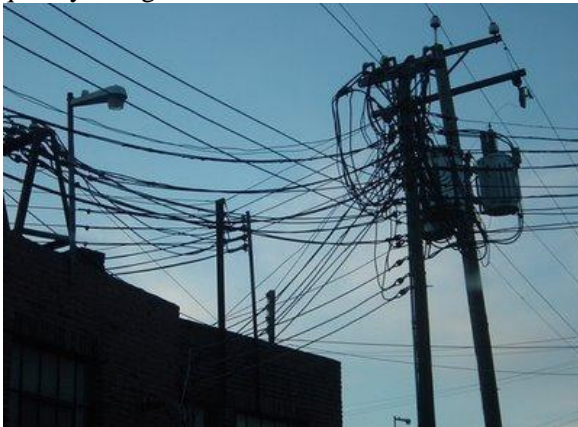
Fig.1 Transmission Line Connection with Wire
