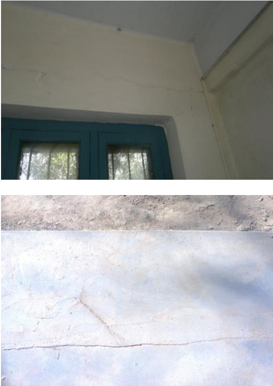
Fig-2 sample cracks appeared in the buildings
